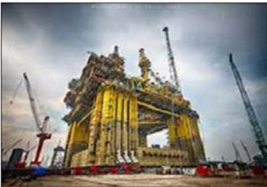
Fig. 11: The semi-submersible FPS for Gumusut-Kakap project (fabricated at MMHE yard, Pasir Gudang Johor, Malaysia (Aug 09-Apr 13)
