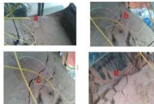
Fig. 12: Failure events before flowslide
