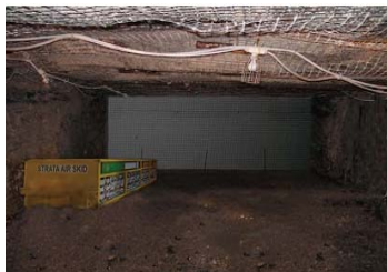
Fig. 2: Arrangement of temporary refuge chamber
