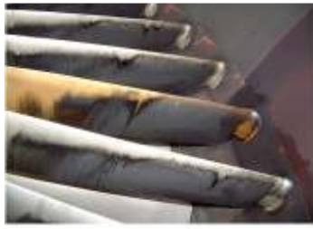
Fig. 3: Fouling on the IGV surface from the gas turbine
