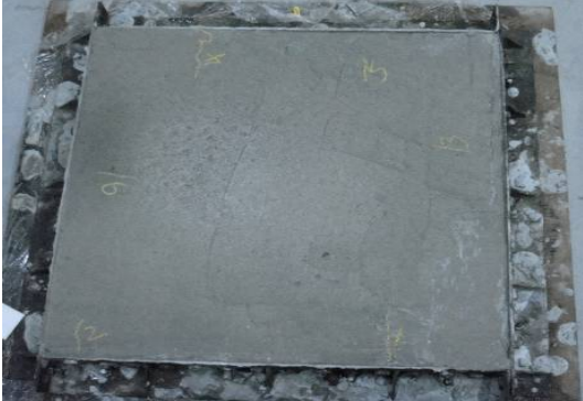
Fig. 3: Cracks in concrete slab
