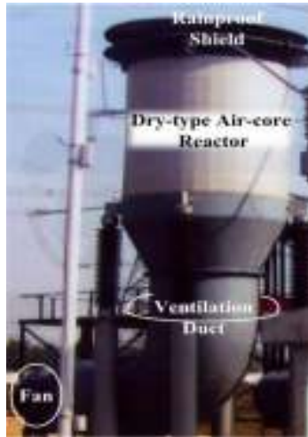
Fig. 1: This type of reactors in substation
