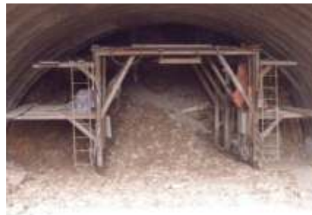
Fig. 1: The collapse of tunnel
