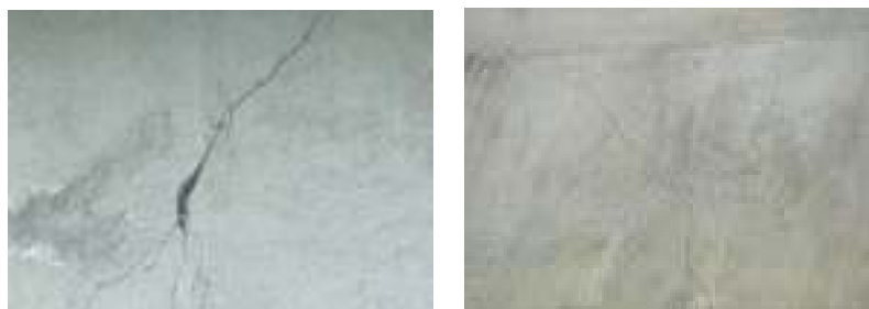
Fig. 2: The cracks in the box girders; (a) outside of box girder, (b) inside of box girder
