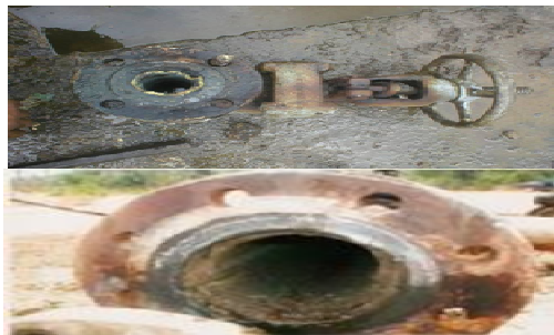
Fig. 3: Scale deposits in pipes and valves (Duccini et al. , 1997)
