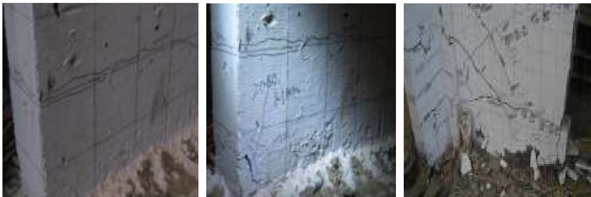
(a) 500 gal cracks of bottom shear wall (b) 2000 gal cracks of bottom shear wall (c) damage of bottom shear wall
