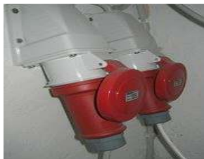
Fig. 14: IEC 60309 style plugs mounted onto a wall socket
