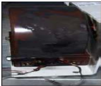
Fig. 3: Burnt damping reactor (ZD) of A-phase for #2 Bus VT
