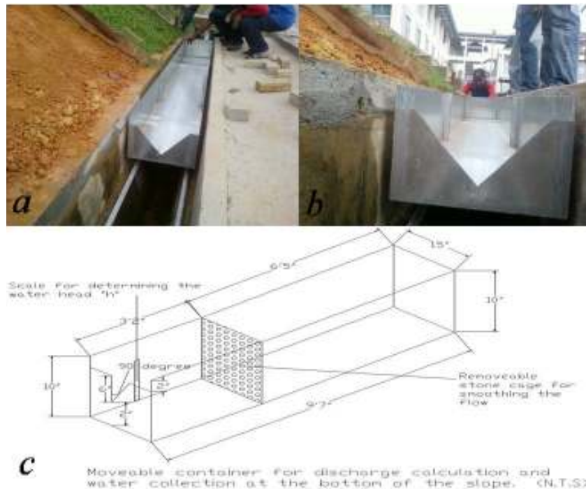
Fig. 9: Details of the bottom container (a, b) bottom container view and (c) detailed drawing
