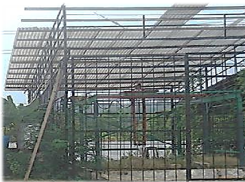
Fig. 7: The shelter-house under study, located at the Universiti Putra Malaysia agricultural experimental field (latitude = 3°0' 9.8094" and longitude = 101°42'11.2926")
