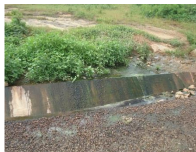
Fig. 5: Leachate seeping from the covered ground
