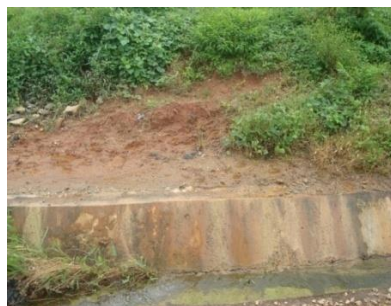
Fig. 6: Leachate seeping to the top soil
