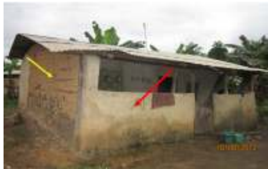
Fig. 4: 12-year old wattle and daub partly rendered with cement mortar (In the construction of wattle and daub, the earth is used in raw form without treatment or additives for the walling: Arrowed yellow is the raw earth material and red arrow shows the cement mortar rendering)
