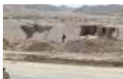
Fig. 10: Slope cut in the wadi bottom and severe gullying, mid-road
