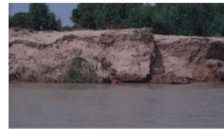
Plate 3: Weakened Channel Bank due to removal of vegetation
